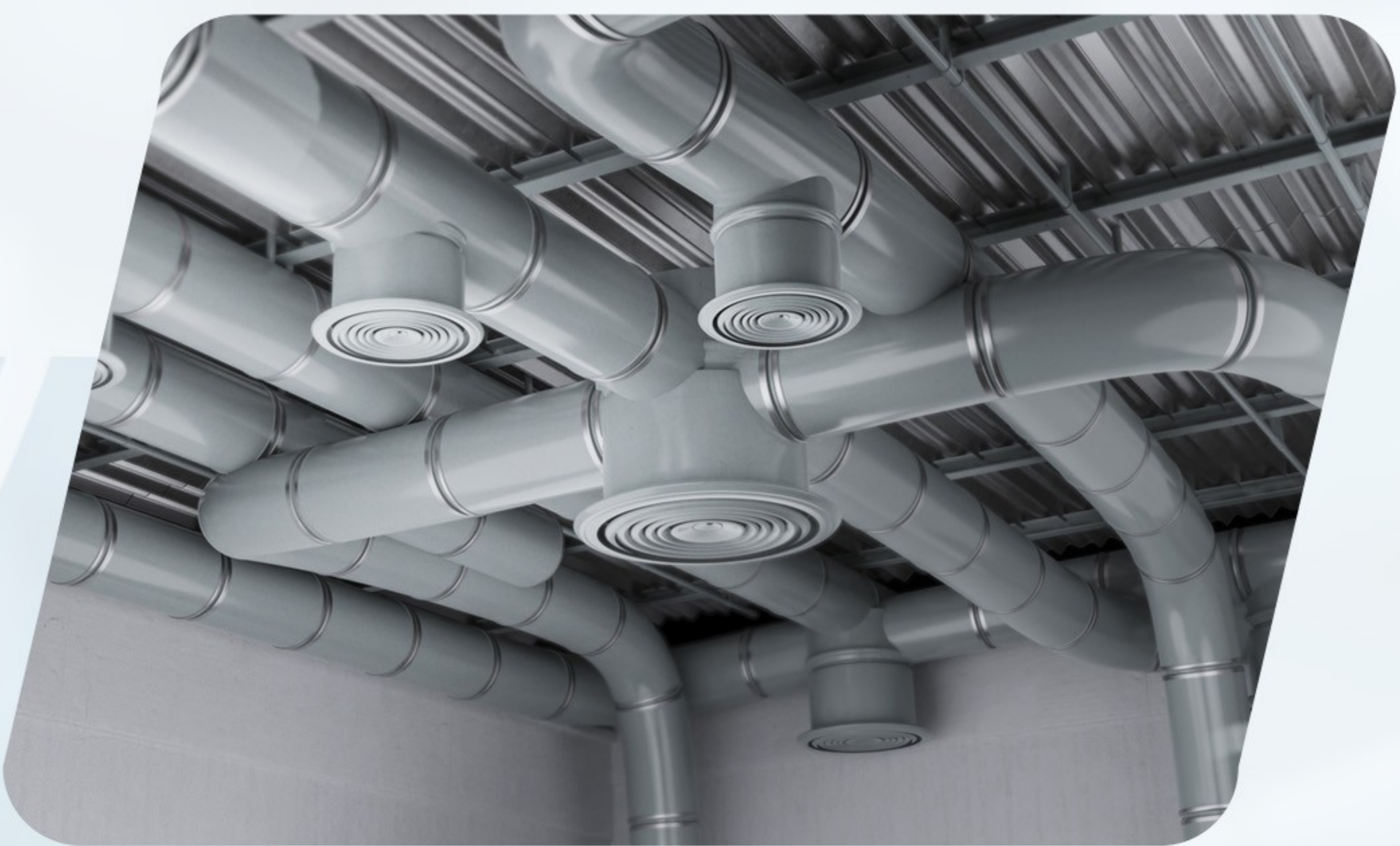
Ventilation & duct pressure monitoring
