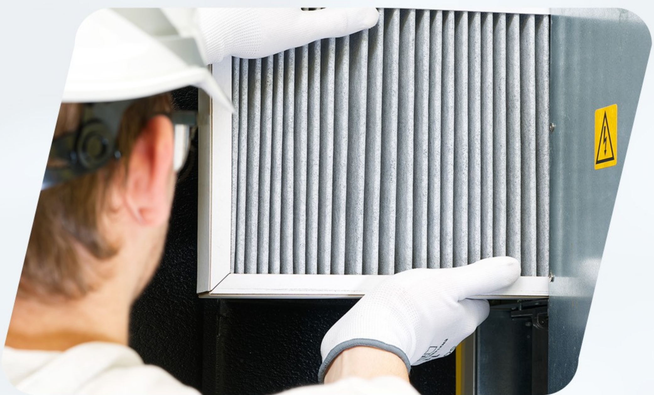
Air filter monitoring (clogging detection)
