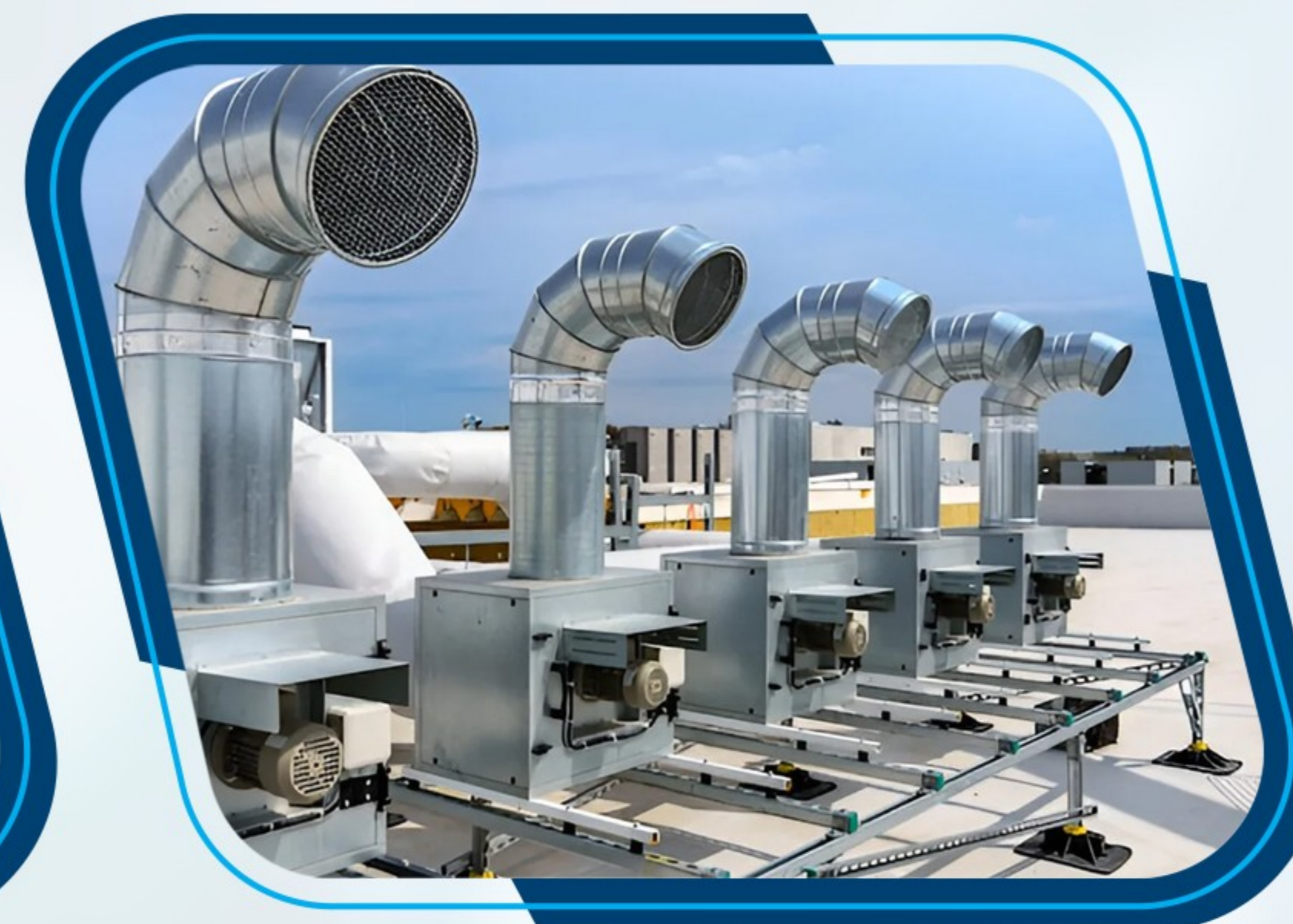
HVAC System Monitoring
