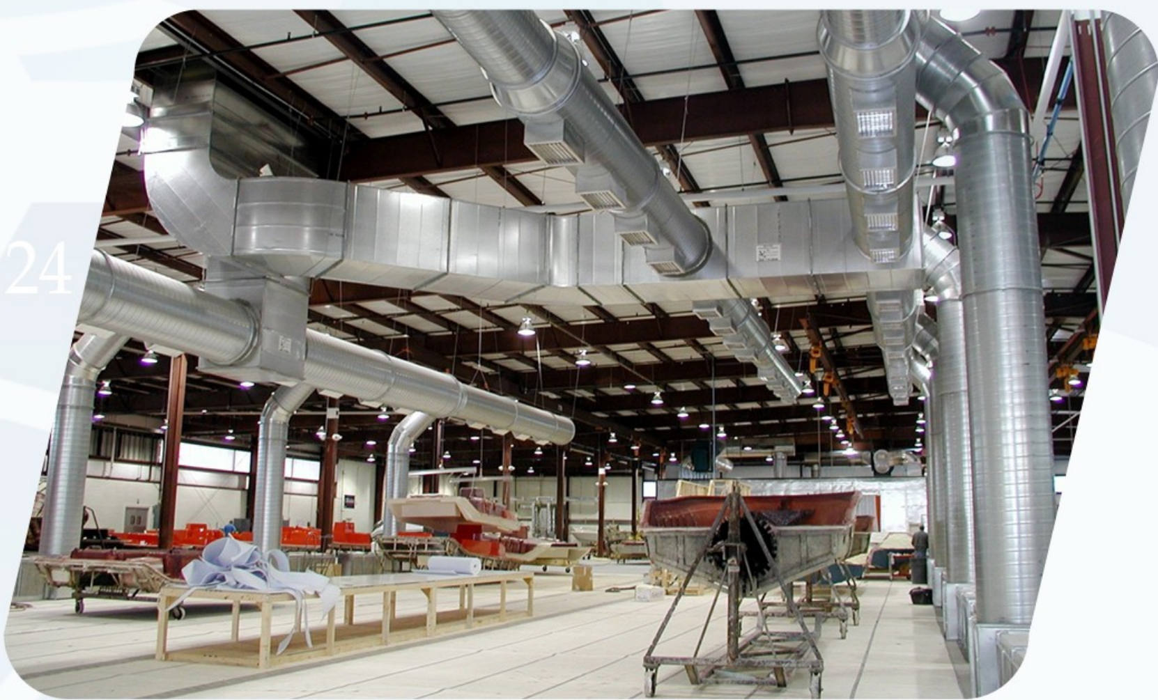
Industrial Ventilation Systems
