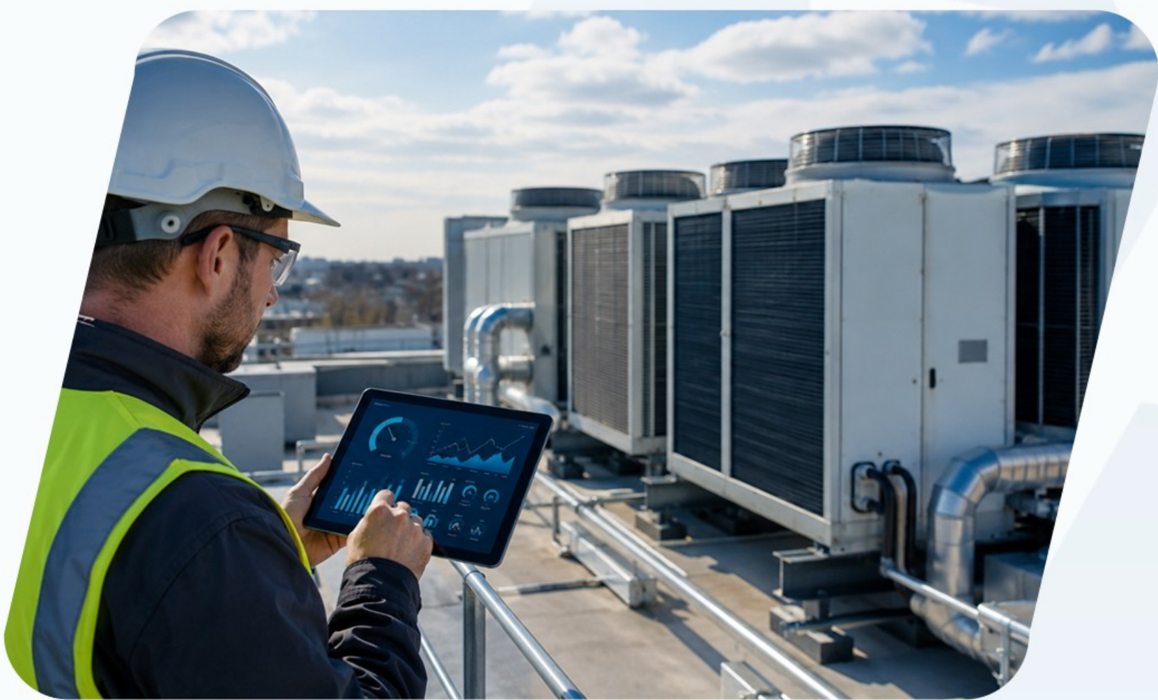
HVAC System Monitoring
