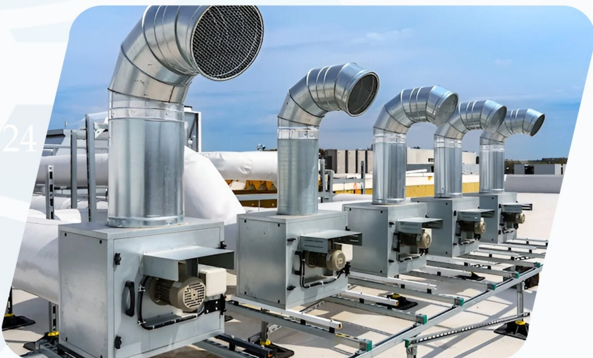
HVAC & Building Automation
