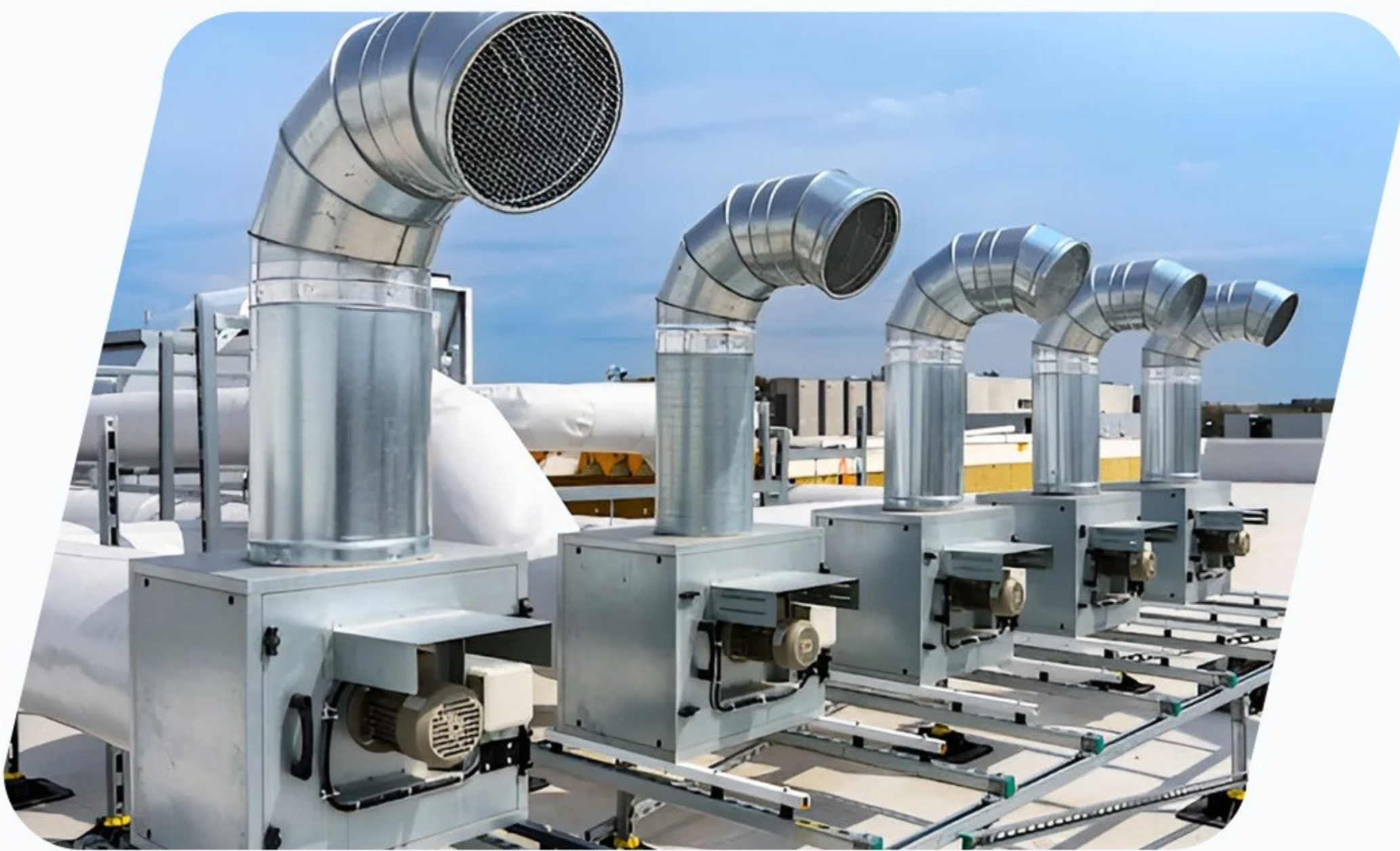
HVAC and Utility Systems
