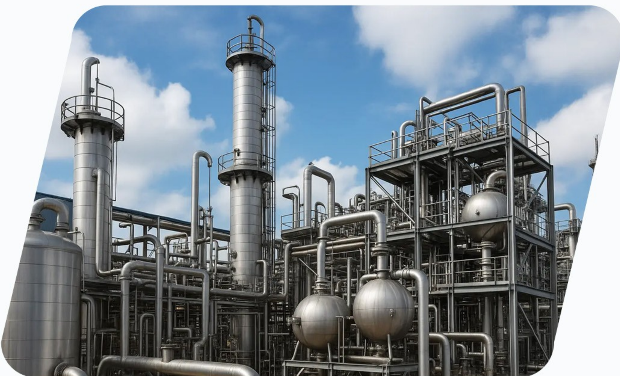
Chemical Industry for Safe Process Temperature Tracking
